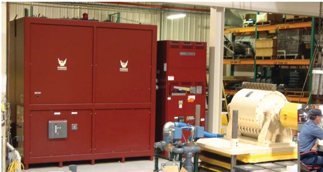
1250 kVA Motor Testing System with Dyno Integration and Remote Control Console.
